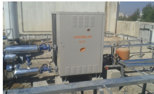
Chiller at Al Balqa
