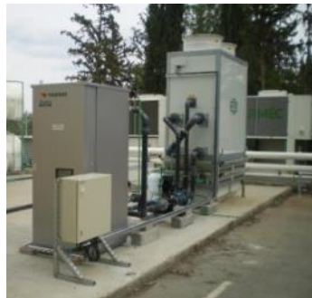
Chiller at Cyl
