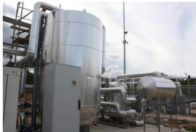
Tank of molten salts (ARCA) and buffer of oil
