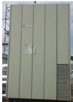
Chiller at ARCA
