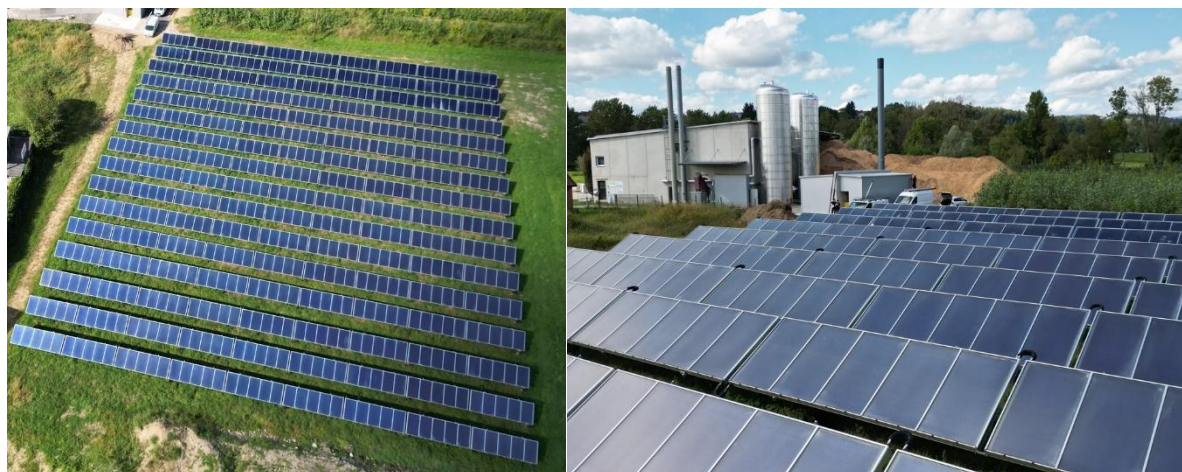
Figure 3. Overview over the installation (left) and overview over the collector field and biomass boiler (right). Source: Nah Wärme St. Ruprecht
