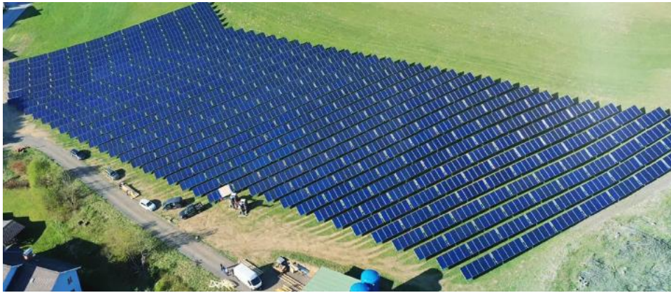
Figure 9. Overview of the installation in Mürzzuschlag. Source: SOLID Solar Energy Systems
