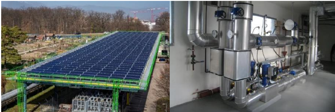
Figure 5. Overview over the installation (left) and the heat transfer station (right) located under the metallic structure.
