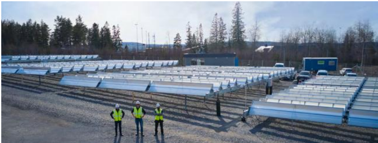
Figure 14. Overview over the installation at Högsletten. Source: Absolicon Solar Collector AB
