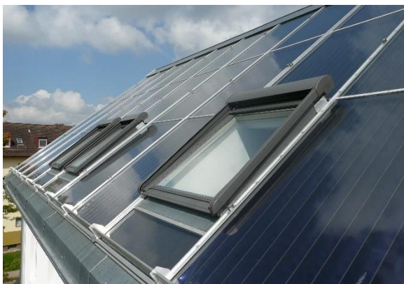
Figure 7: Roof integrated solar thermal collectors on “solar@home”-building in Crailsheim, Germany (Solites)
