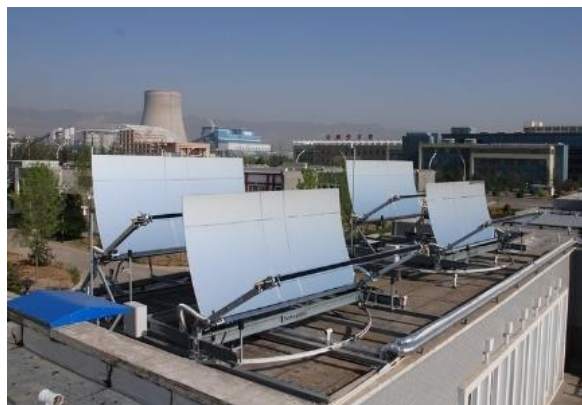
Figure 8: Demo system of Sun Oyster on a flat roof in Zhangjiakou, China (sunoyster.com)
